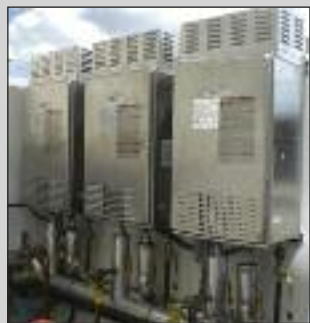
Noritz N-1321M-ASME commercial tankless water heaters supply endless hot water to 208 guest rooms in a California hotel.
